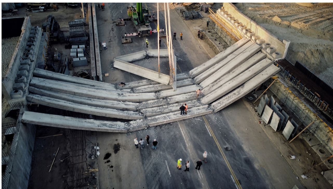
Complex undertaking: a road bridge under construction in Kyiv. © Yan Dobronosov/Global Images Ukraine via Getty Images
