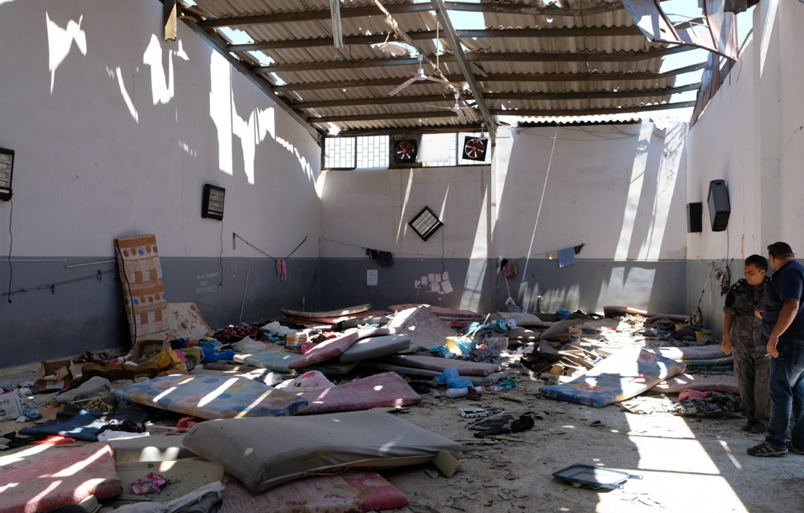
The main dormitory of the Tajoura detention centre after having taken the blast from an airstrike on an adjacent building on 2 July 2019. © Mark Micallef
